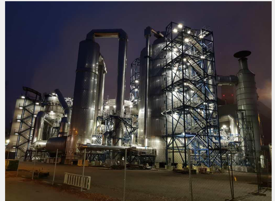
Acid plant Harjavalta
