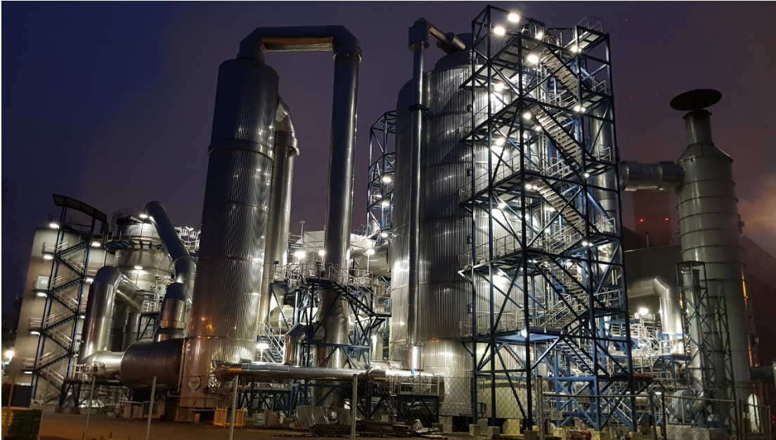
Harjavalta acid plant
